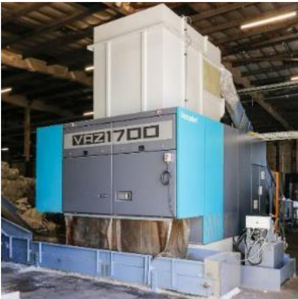
Photo 1: The Vecoplan VAZ1700 installed at YS Reclamation
